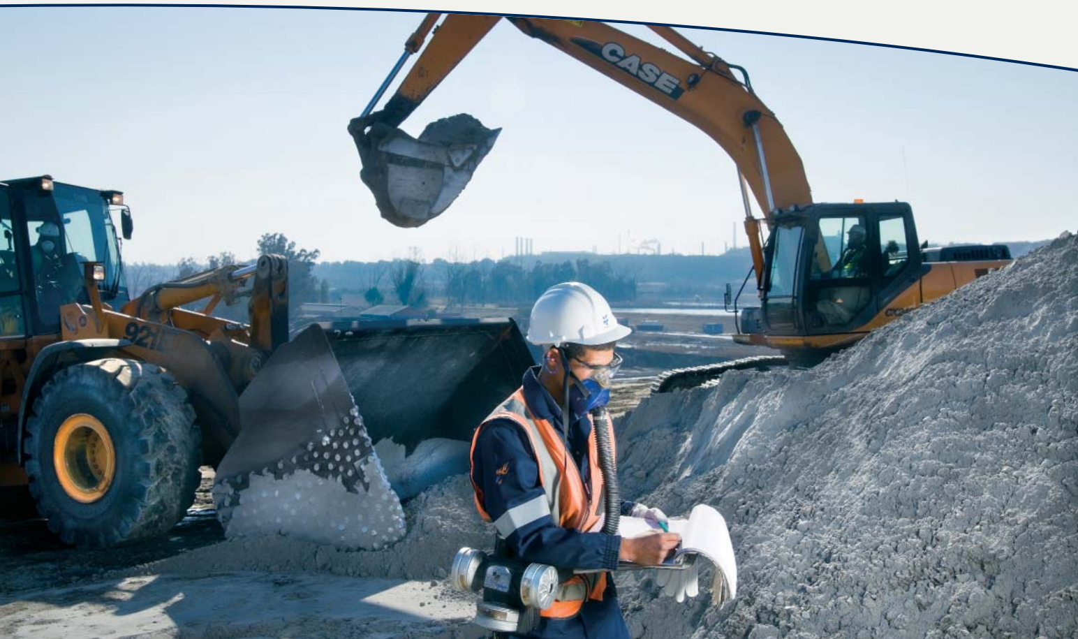
Huyan Allie keeps records of loads of ash to track and control blending ratios at the tarpit blending project at Sasolburg, where fine and coarse ash are blended with tar to stabilise the tarpits.
